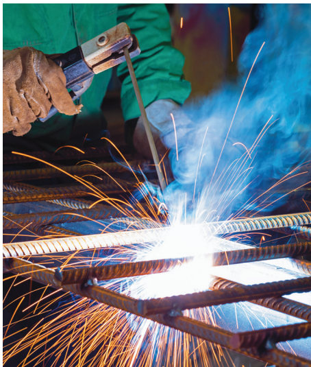
Suction of welding fumes
