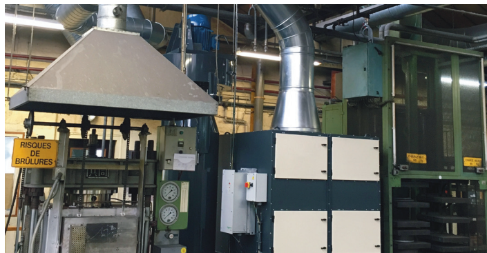
Extraction of metallic dusts on sintering press. Filtration with FILTRACLEAN ECO
