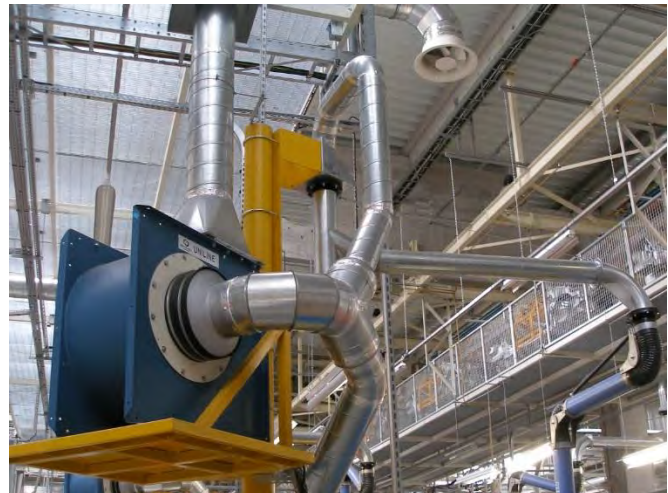
Extraction of welding fumes
