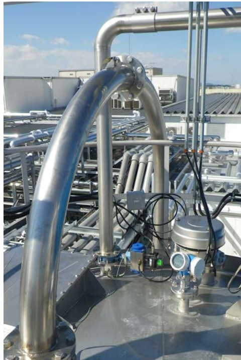
Silo feed pneumatic conveying
