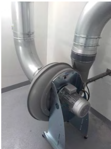
Extraction of steam
