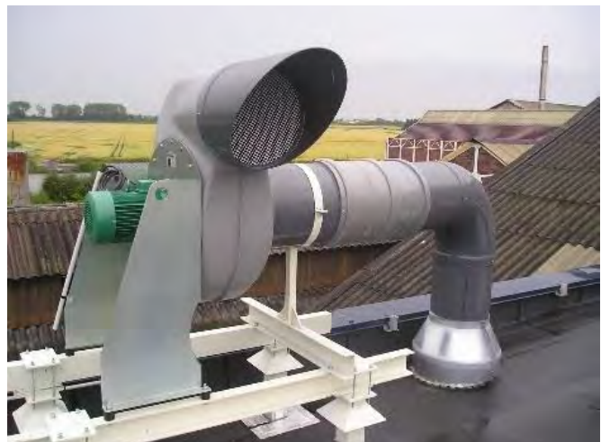
Extraction of corrosive gases
