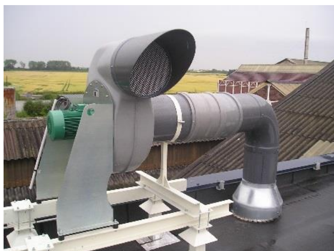
Extraction of corrosive gases
